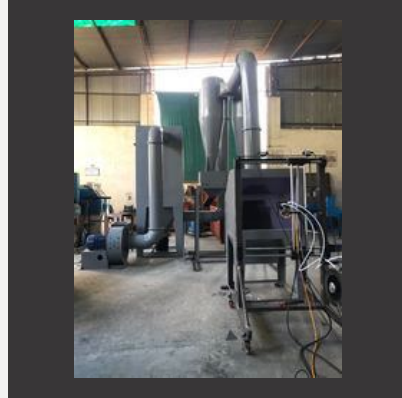
Metallizing Spray Booth
