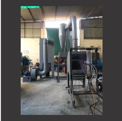
Metallizing Spray Booth
