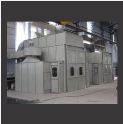
Paint Spray Booths
